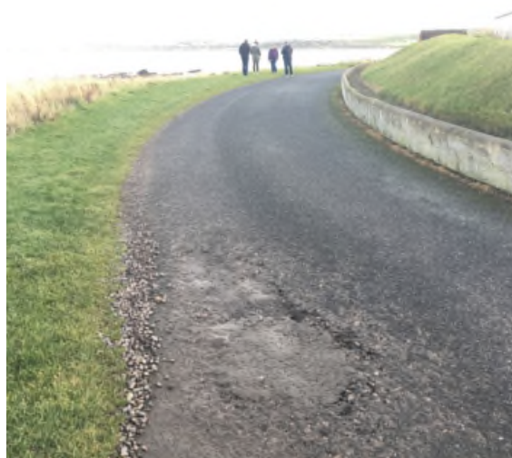
Figure 1 Road width and damage to edge of road carriageway
